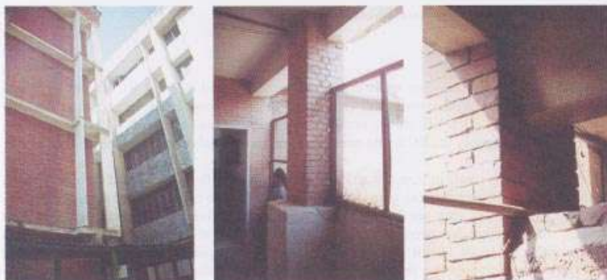
"L" building: Left: Masonry or RC blocks can fall down and injure people during a MMI = VI-VII earthquake. Middle and Right: Short columns will be able to trigger the building and lead to fragile-collapsing-mechanism (pancake failure) during a MMI = VII earthquake.
