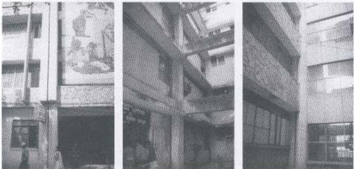
"New" buildings. Left: Seismic joint of small size in the main building facing Kanti Path. Middle: Diaphragm discontinuity in one of the three structures composing the main new building. Right: Masonry parapets rigidly connect the new buildings where a seismic joint was designed.
